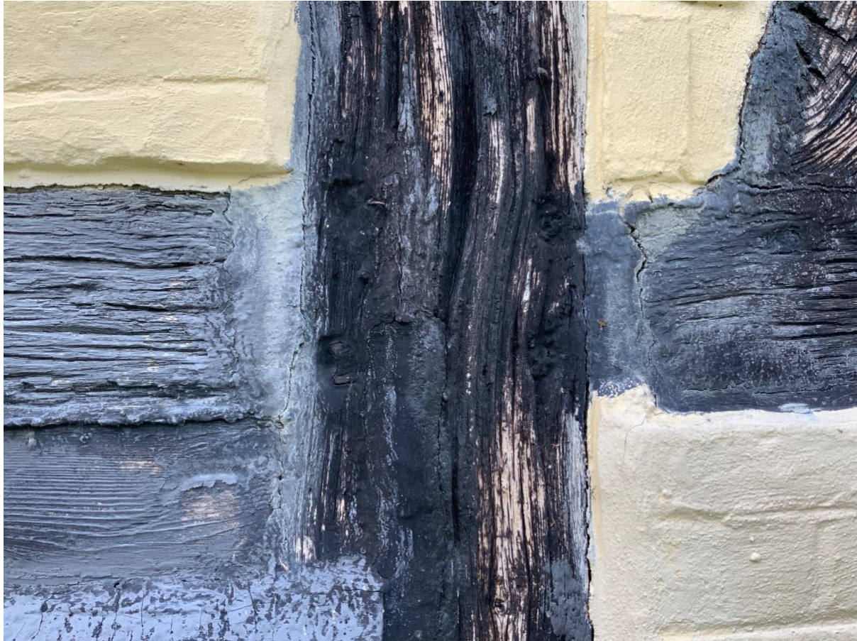
Figure 16, impervious paints and filled joints.
