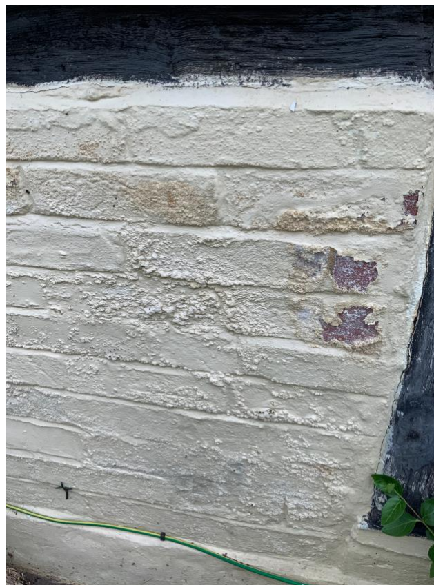
Figure 18, Blistering impervious paint.
