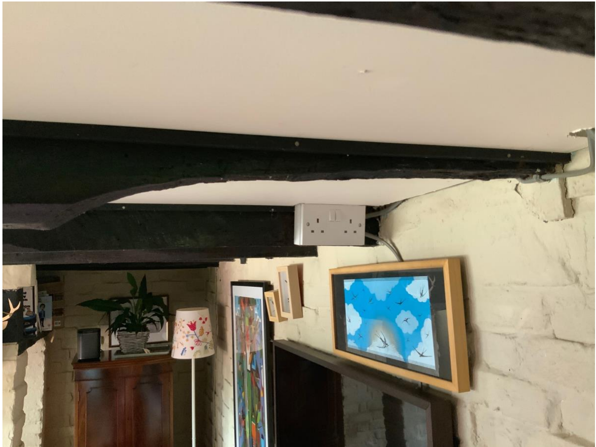
Figure 15, Joists cut away to accommodate a tall piece of furniture.
