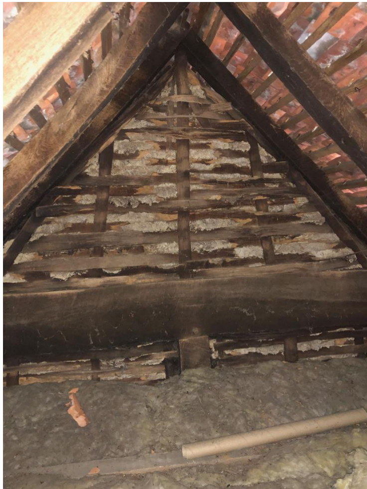
Figure 22, View of cross-frame II from inside the neighbouring bay roof space. (Author 2019)
