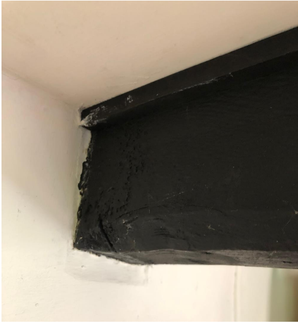
Figure 9, Joist end showing chamfer stop. (Author 2019).
